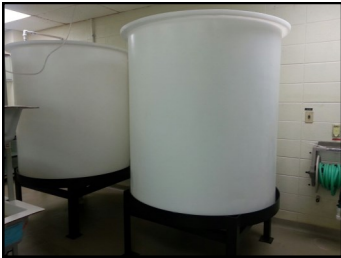
New water storage tanks
